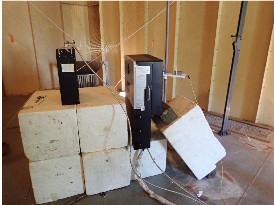
Test Setup of EG 4LL100Ah Server Rack (Serial No. SC2022101794) and EG4 18kPV Hybrid Inverter (Serial No. 3464660222) on Z Axis
