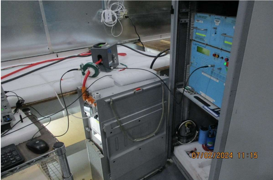
Test Setup for CS117, Actual Test Waveform #2 & #3 on Battery High Side
