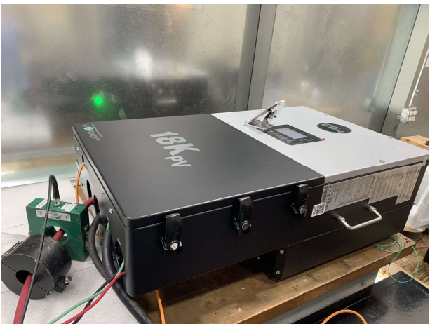
CS116 Test DC High Side
