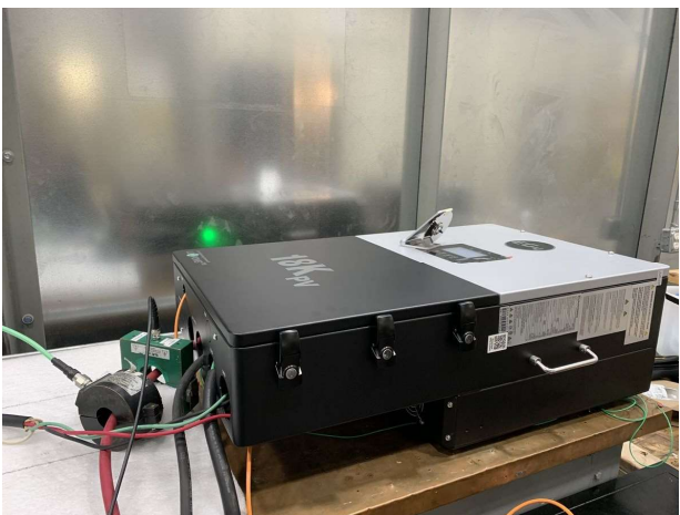
CS115 Test DC High Side
