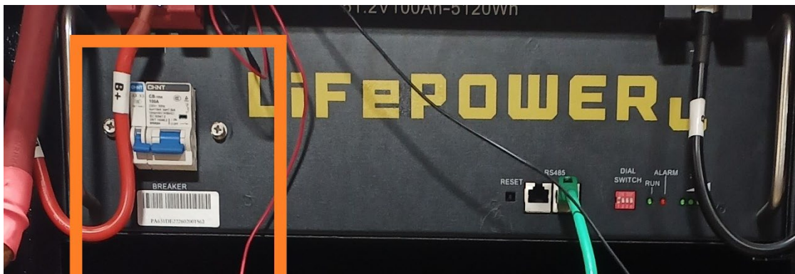
Battery circuit breaker OFF
